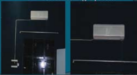
Air conditioning system
